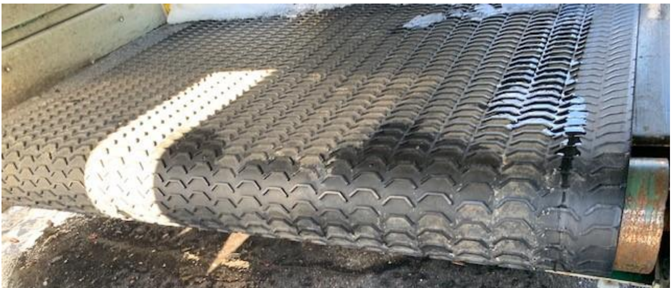
Conveyor 19-294 with Shredder 19-293
